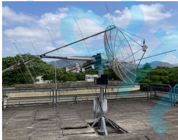
Figure 12: VHF and UHF Antennae positioned in the Roof of the Southern Space Coordination of the National Institute for Space Research – COESU/INPE – MCTI, in Santa Maria, RS.
