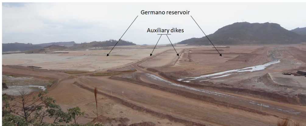
Fig. 17 Field picture of the auxiliary dike and the reservoir in the Germano mining complex.
