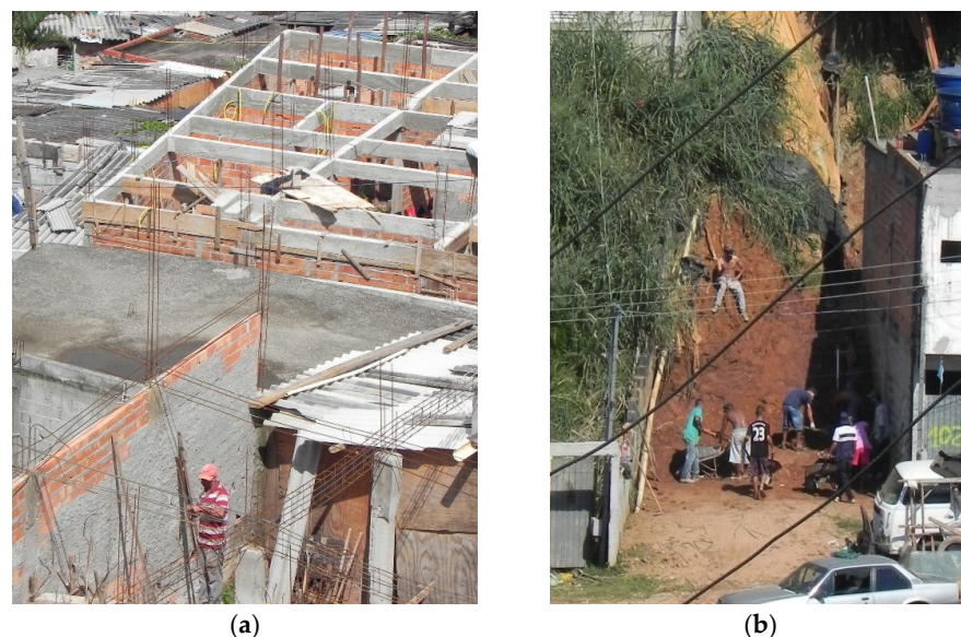
Figure 2. Common self-aided practices in informal settlements: (a) building houses; (b) terrain cut.
